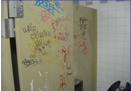
Men's bathroom during initial CORE visit
